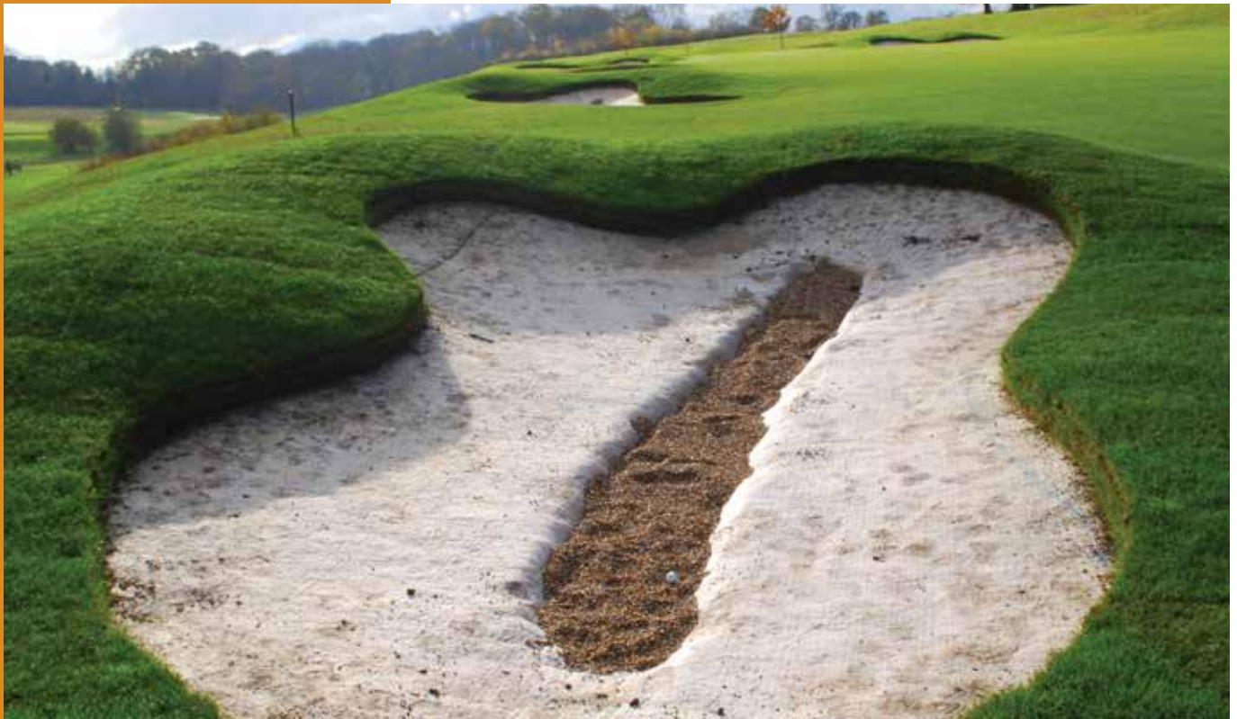
BEACHED BALL The HyLine Bunker Liner, complete with drainage channel, before sand is installed
